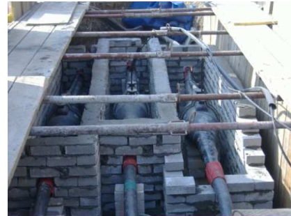
Figure 4: Example of a 400 kV joint bay directly buried into the ground; Typical dimension: length 10 m, width 2.5 m, depth 2.1 m
