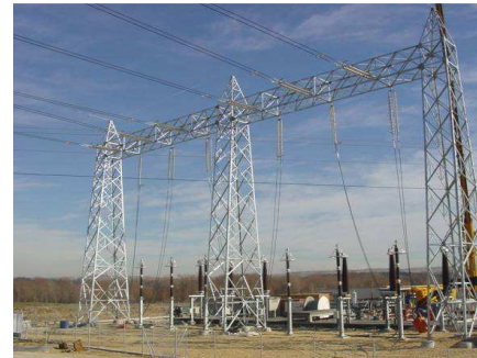
Figure 5: Overhead line cables transition station (400kV)
